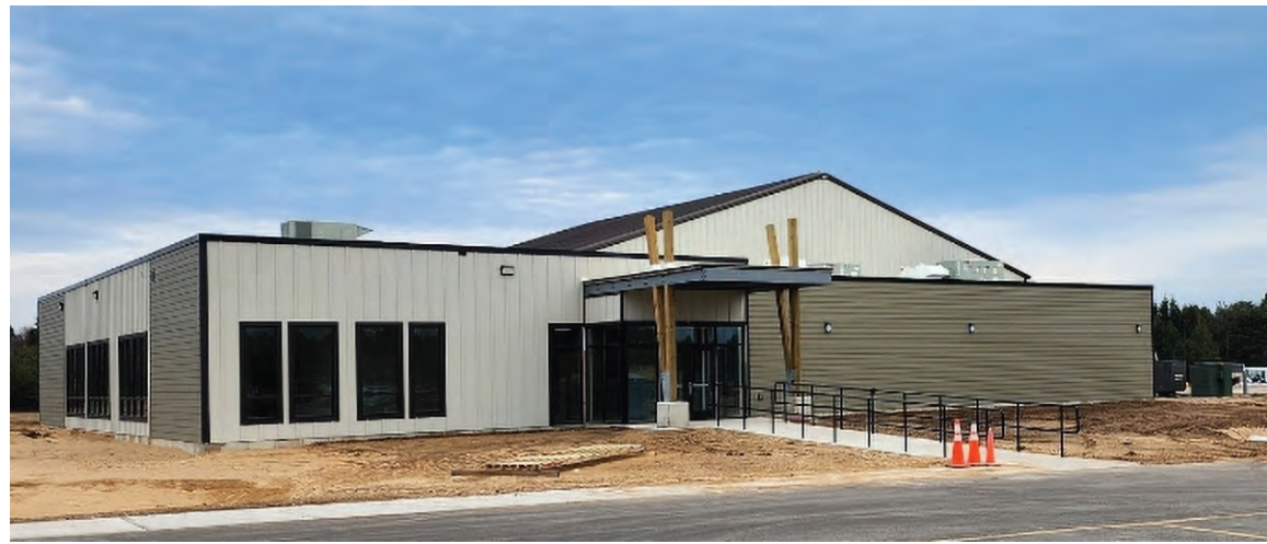
Manistique's new fitness center under construction is next to the health center.
