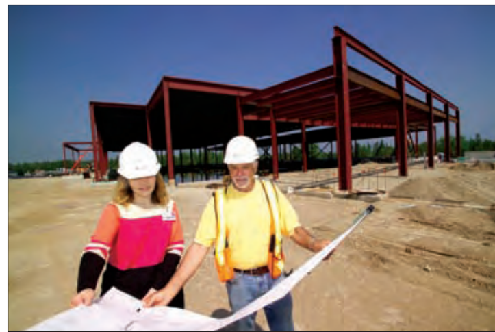
The structure takes shape. Darcy Chase, manager of the Kewadin Shores Casino and Lenny Adams, project site manager, look over the blueprints with the steel I-beam frame of the new Kewadin Shores rising behind them.
