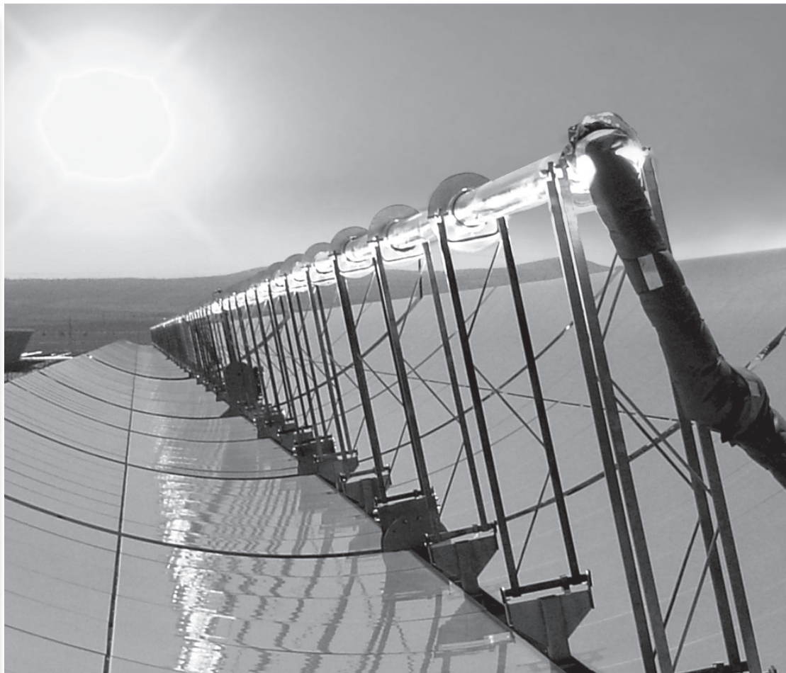
Concentrated solar power
