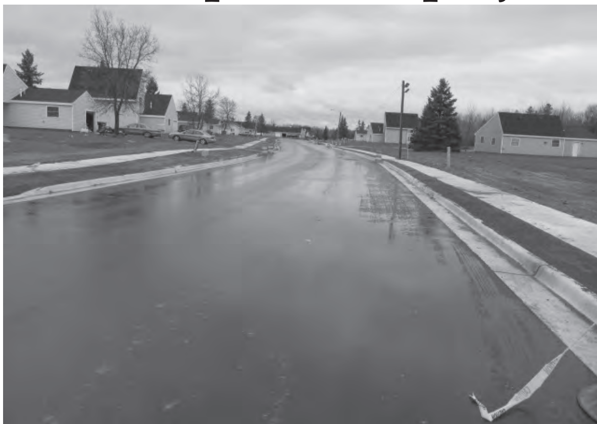
Photo Courtesy Wendy Hoffman Reconstruction of Shawano Drive and cul-de-sacs along with installations on Ice Circle Drive was the major construction project for 2014. The project was completed with some restoration (seeding) to be finished in the early spring of 2015. The project addressed numerous structural deficiencies in drainage, pavement, pedestrian mobility and safety.
