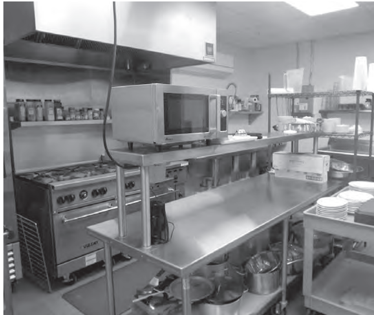
Hessel kitchen area after renovations. The new area boasts a larger and range and oven, refrigeration, walk-in cooler and freezer.
